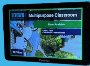
INSTALLED ROOM OCCUPATION DISPLAYS TO REDUCE PAPER USAGE AND REFLECT REAL-TIME CHANGE
