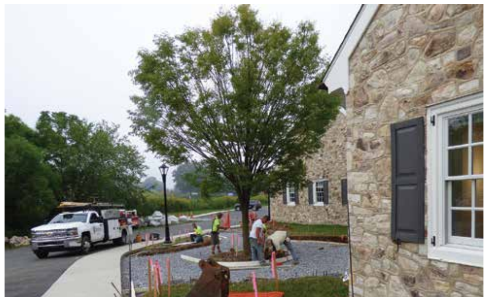
Workers install a patio and garden near the Young Center's new front entrance.
