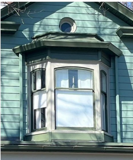
Located on the second floor is a Canted Bay Window. Directly above the window is an oculus window.
