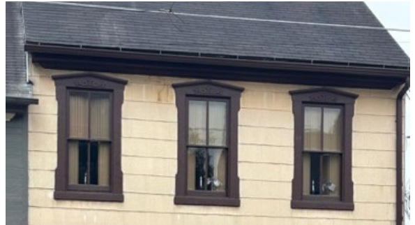
Double hung windows, two over two panes separated by thin wooden muntins. Victorian
