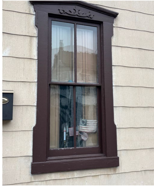
Wooden lintels, not flat but coming to slight peaks at centers with more delicate molding
